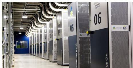
Harding Street Station storage facility | AES
